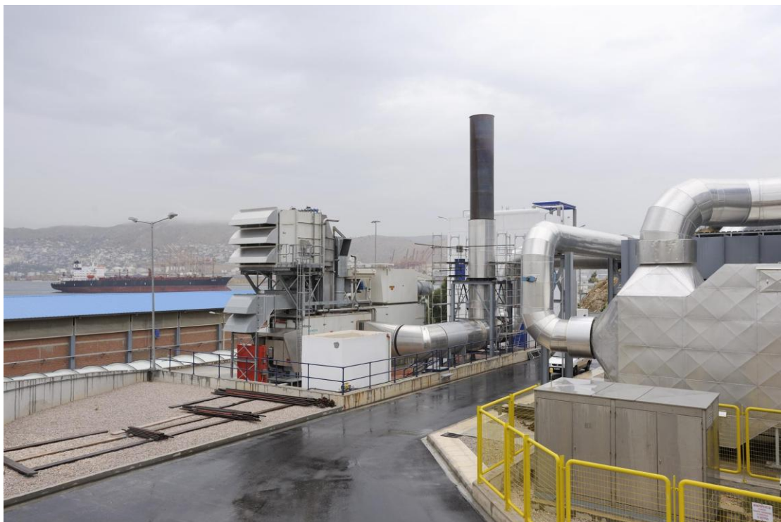
Picture 1 Siemens SGT-400 Gas Turbine generator (14 MW) set in Cogeneration application at Psyttalia - Sewage Treatment Plant - Greece
