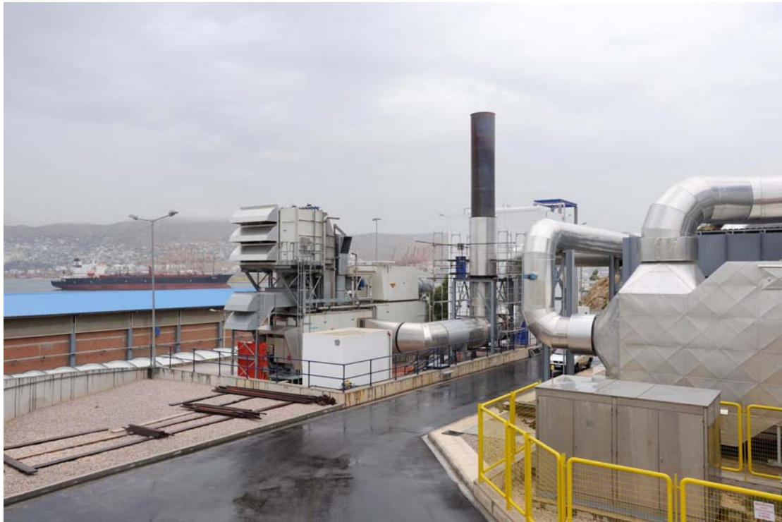
Picture 1 Siemens SGT-400 Gas Turbine generator (14 MW) set in Cogeneration application at Psyttalia - Sewage Treatment Plant - Greece
